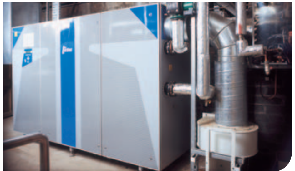
CHP Plant with Heat Exchange Unit
