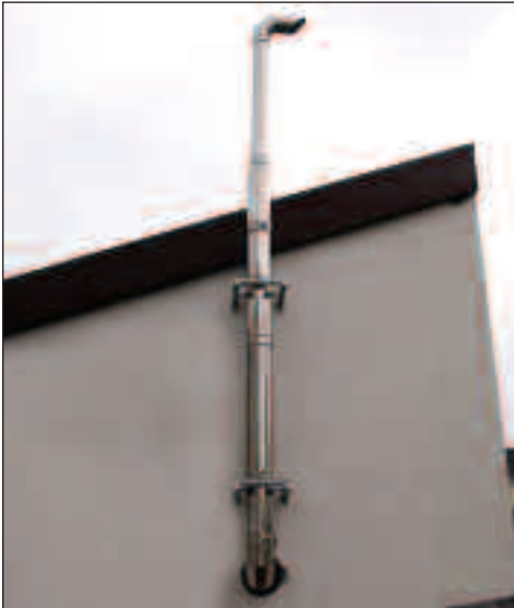
The flue from the CHP plant, Clybaun Hotel.
