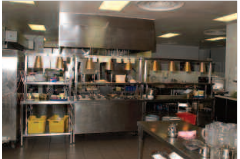
The full service kitchen at the Clybaun Hotel.
