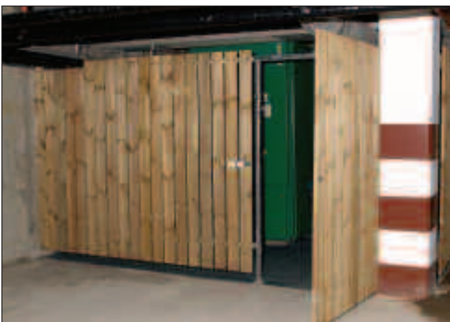
The CHP unit partitioned in the naturally ventilated basement car park, Clybaun Hotel.
